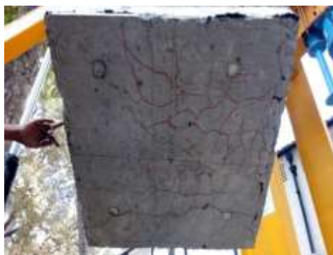
Fig. 12: Cracks on the slab after loading
