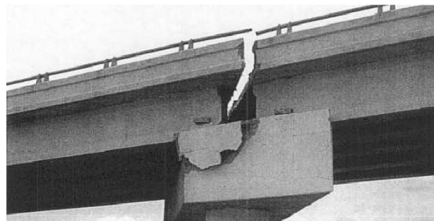
[Fig.3: Cracks in Skew Bridges Due to Earthquake [12]]
